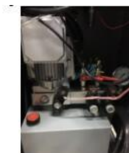
Picture 27 (oil tank)
